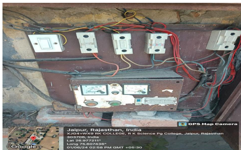
Motor Starter Panel
