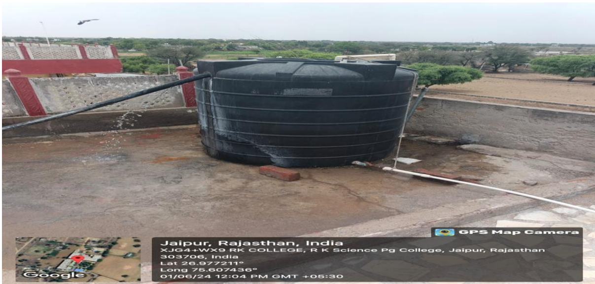
Water tanks present in college
