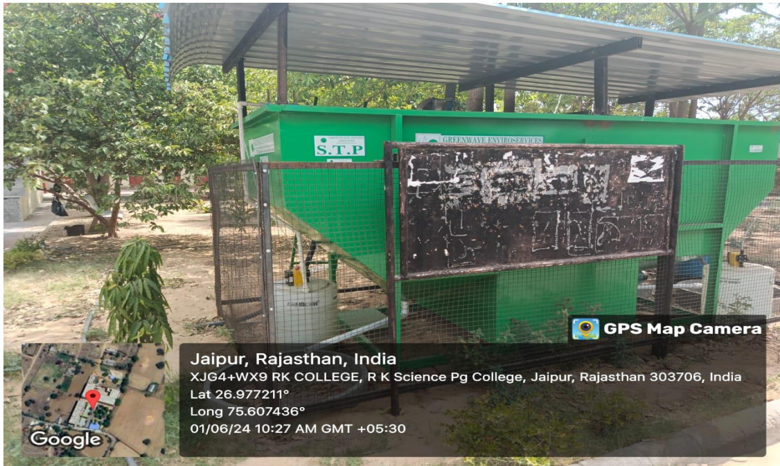
Sewage Treatment Plant (if present)
